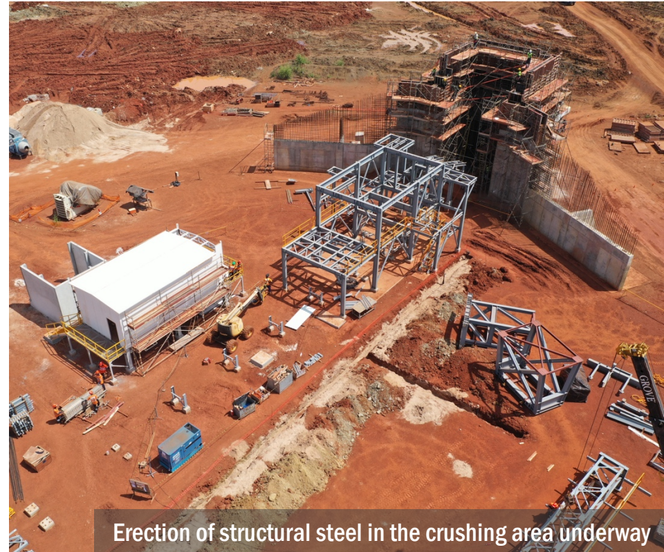
Erection of structural steel in the surge bin area; assembly of the mill feed conveyor underway
