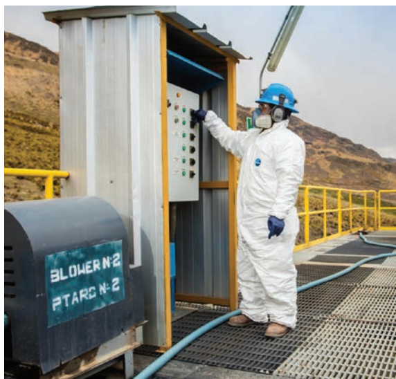
Caylloma Mine water treatment operation panel
